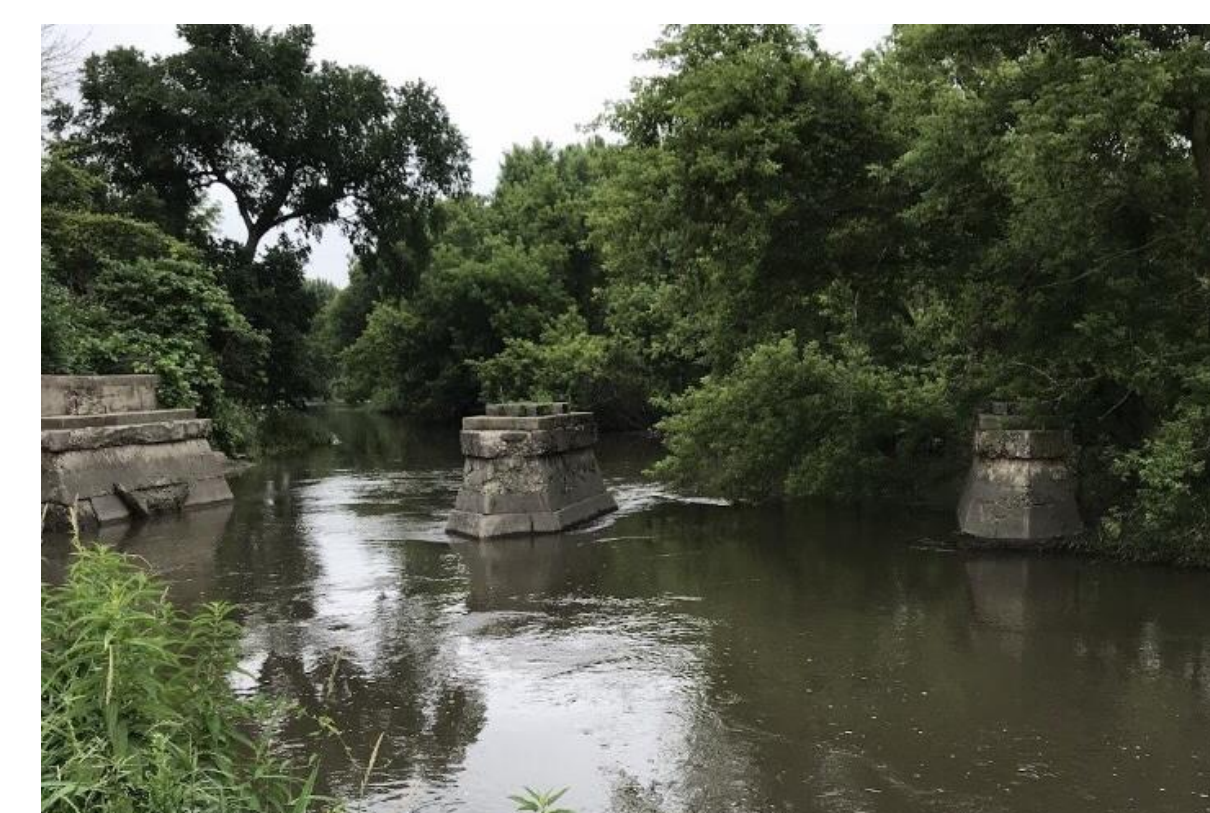
Fig. 8. Broken Bridge Summer
