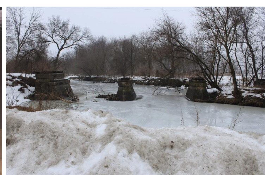
Fig. 3. Broken Bridge Winter
